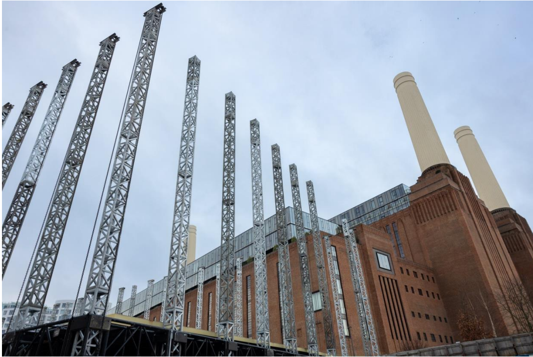
Caption: Construction is well underway on NEON at Battersea Power Station, which will open in Spring 2025 Image credit: Star Live
